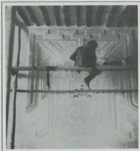
House restoration in Shela, Kenya, Aga Khan Program Archives, donated by James de V. Allen
