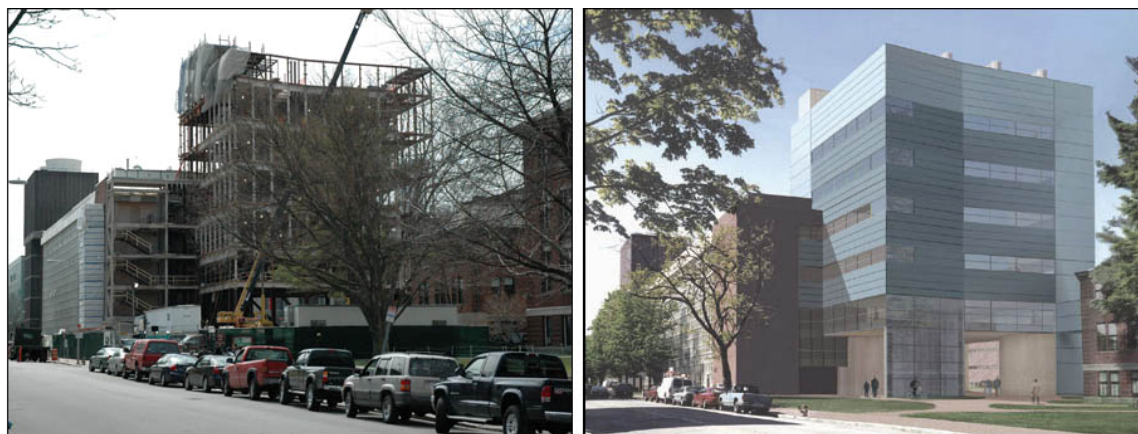
Figure 10.1. Construction underway at Harvard University (left) on the new Laboratory for Integrated Science and Engineering (LISE), April 2006. Computer aided design of the completed LISE building (right) that will be the new home of the shared experimental facilities.
