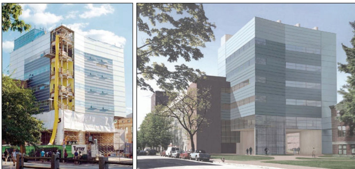
Figure 10.1. Construction nears completion at Harvard University ( left ) on the new Laboratory for Integrated Science and Engineering (LISE), November 2006. Computer aided design of the completed LISE building ( right ) that will be the new home of the shared experimental facilities.
