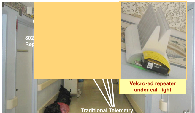
Fig. 6. Repeaters were attached to call lights at the step-down unit hallway of the Washington Hospital Center.
